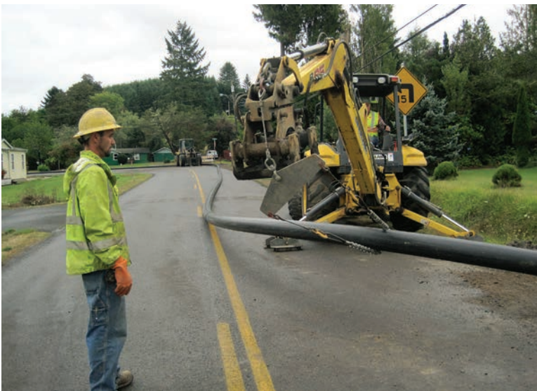
K&R Plumbing employees Brandon Moore (left) and Steve Roberts guide 8-inch HDPE pipe into a pipe bursting machine.
