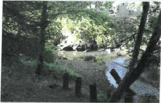
4. Significant bank erosion
