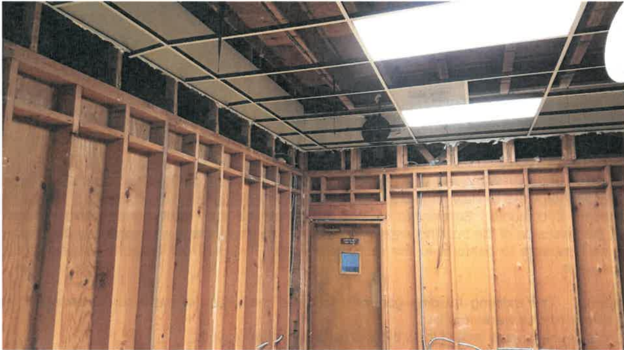
Interior shear wall sheathing does not continue to flat roof.
