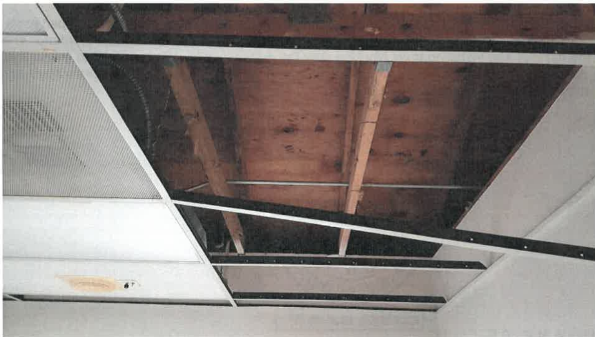
Truss blocking over exterior shear walls not present.
