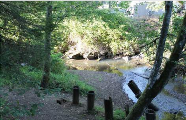
4. Significant bank erosion
